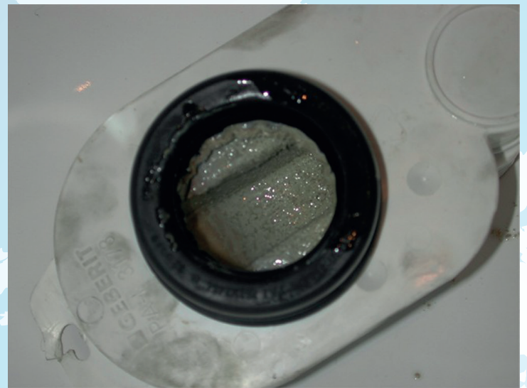
Siphon before use of Cee-Bee™ MR Vacuum Toilet System Cleaner
